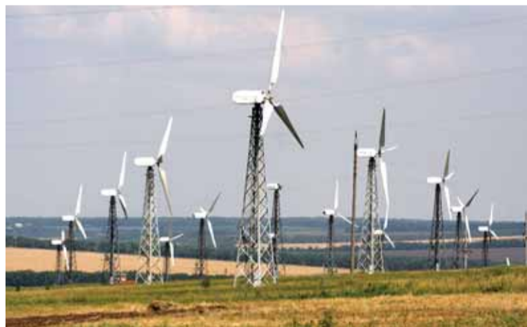
Wind-based electricity making is a part of Ukraine's $3.7 billion alternative energy market. Photo taken at Novoazovsky wind park in Donetsk Oblast on July 11, 2011. (PHL)
