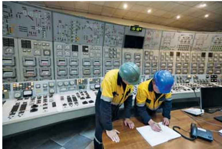
Workers at the Kyiv-5 heat energy plant in August 2014. Naftogaz envisions building two new, more efficient power plants in Kyiv with the Chinese loan. (Volodymyr Petrov)
