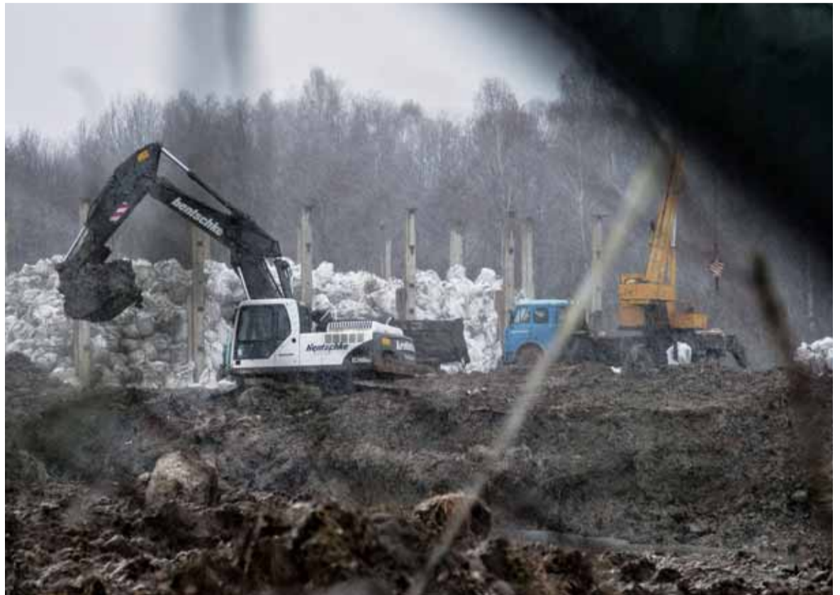
An excavator which belongs to SI Group company takes the bags with hexachlorobenzene from the polygon of chemical waste in Kalush, Ivano-Frankivsk Oblast on November 25, 2013.
