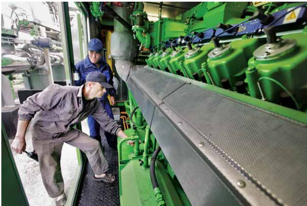
Workers check the control system of one of two generators operating at the Rokytno biogas plant. Within the generator, internal combustion engines generate electricity from biogas. (Pavlo Podufalov)
