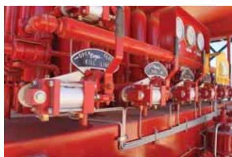
BOP Control System of OCO (USA) used for well sealing, fire and pollution prevention
