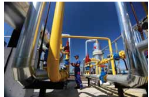
Working well near “Zhuravlyna” gas preparation unit (GPU)
