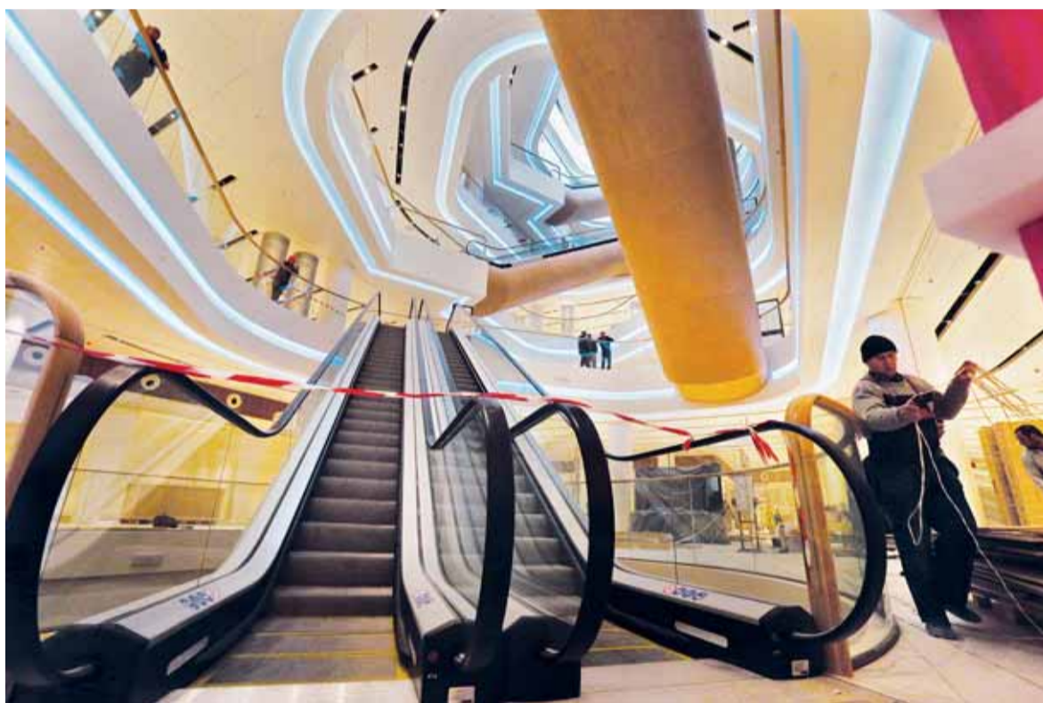
A man works in the TsUM store during the reconstruction on Oct. 26. (Volodymyr Petrov)
