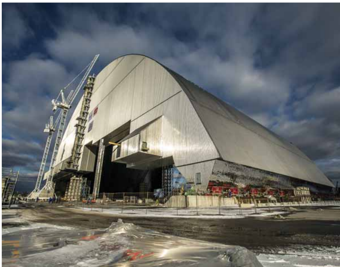
The Chernobyl nuclear power plant's safe confinement arch is 165 meters long, 110 meters high and weighs more than 36,000 tons. It is made by the French construction consortium Novarka. The process of covering of the fourth reactor began on Nov. 14. (Courtesy by EBRD)
