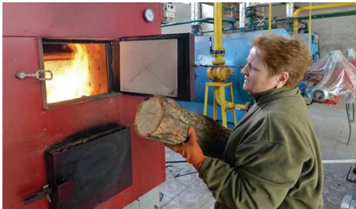
A worker loads firewoods in a boiler in the western Ukrainian town of Zolochiv on Oct. 28. The administration of the 25,000-resident city of Zolochiv, some 60 kilometers from Lviv, rejected the use of gas for heating and completely switched to an alternative fuel – wood. (AFP)
