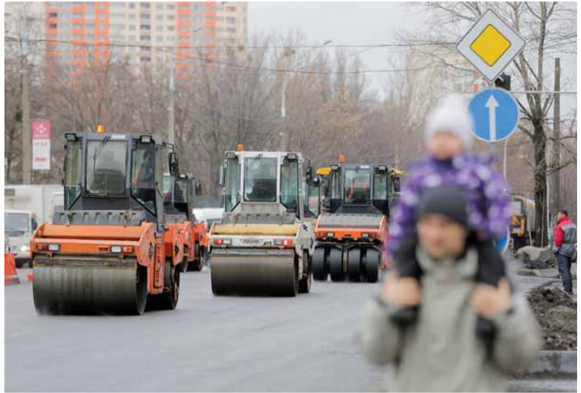
A fleet of steamrollers flatten a surface of a repaired road in Kyiv on Dec. 10. For 2018, the Ukrainian government has allocated $1.8 billion to renovate the country's 169,500-kilometer road network. (Volodymyr Petrov)
