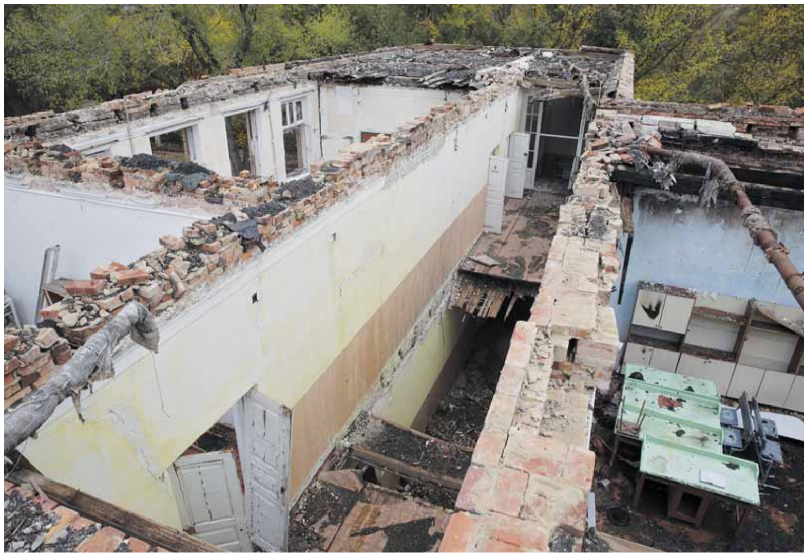
The remains of a destroyed public school in the war front city of Krasnohorivka, a Ukrainian-controlled Donetsk Oblast city of 15,000 residents some 560 kilometers southeast of Kyiv, on Oct. 11. (Volodymyr Petrov)
