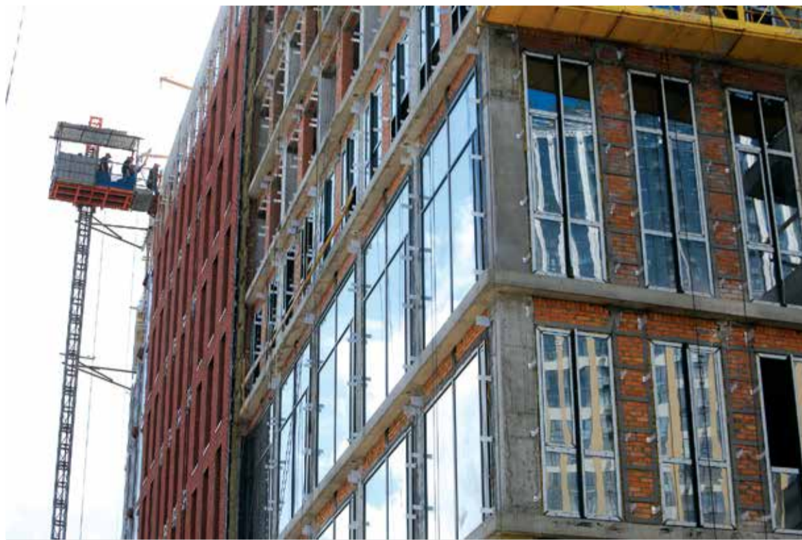
A construction team works on Chicago, a residential complex under construction by Saga Development, in central Kyiv on May 21, 2018. (Volodymyr Petrov)
