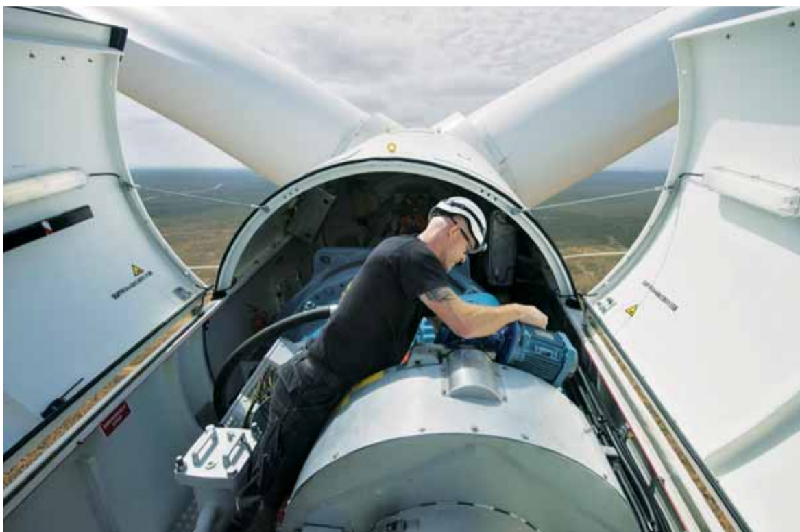
Siemens engineer Danish Lars Birkmann works on a Siemens wind turbine on Nov. 6, 2015. (AFP)
