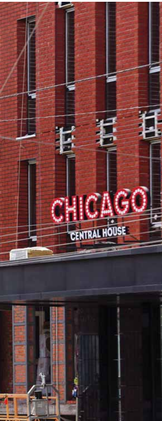
Workers get a lift to build Chicago, (right) a new apartment development in downtown Kyiv. Chicago is meant to attract clients with a bohemian, extroverted outlook, says its developer, Saga Development. It's one of a slew of new developments that's using American names to sell real estate near Kyiv. (Volodymyr Petrov)
