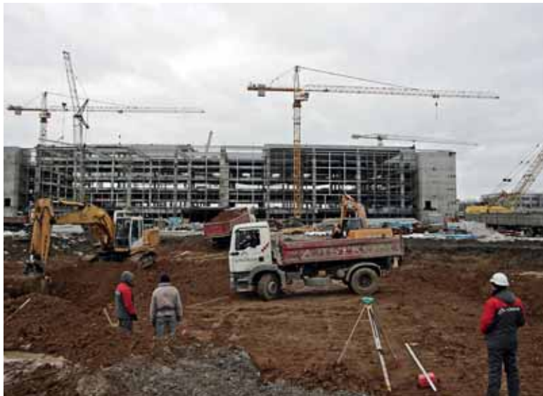
Workers from Altcom take part in construction of a new airport in Donetsk on Feb. 9, ahead of the Euro 2012 football tournament which is being co-hosted by Ukraine and Poland. Four cities in each country are hosting games. Ukraine's capital, Kyiv, is hosting the final on July 1. (AFP)
