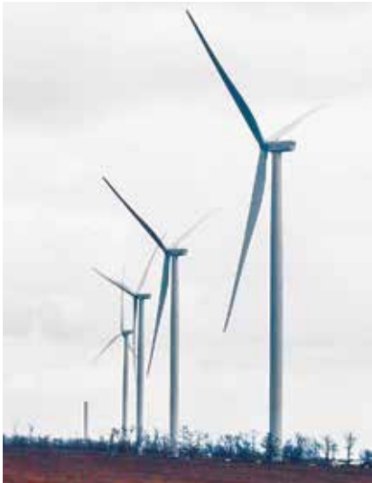
Turbines rise above trees at Primorskaya wind farm in Zaporizhia Oblast. The installation was one of many renewable energy projects launched in 2019 as developers race to grab the last of Ukraine's generous feed-in tariff. (Mykola Lazarenko)
