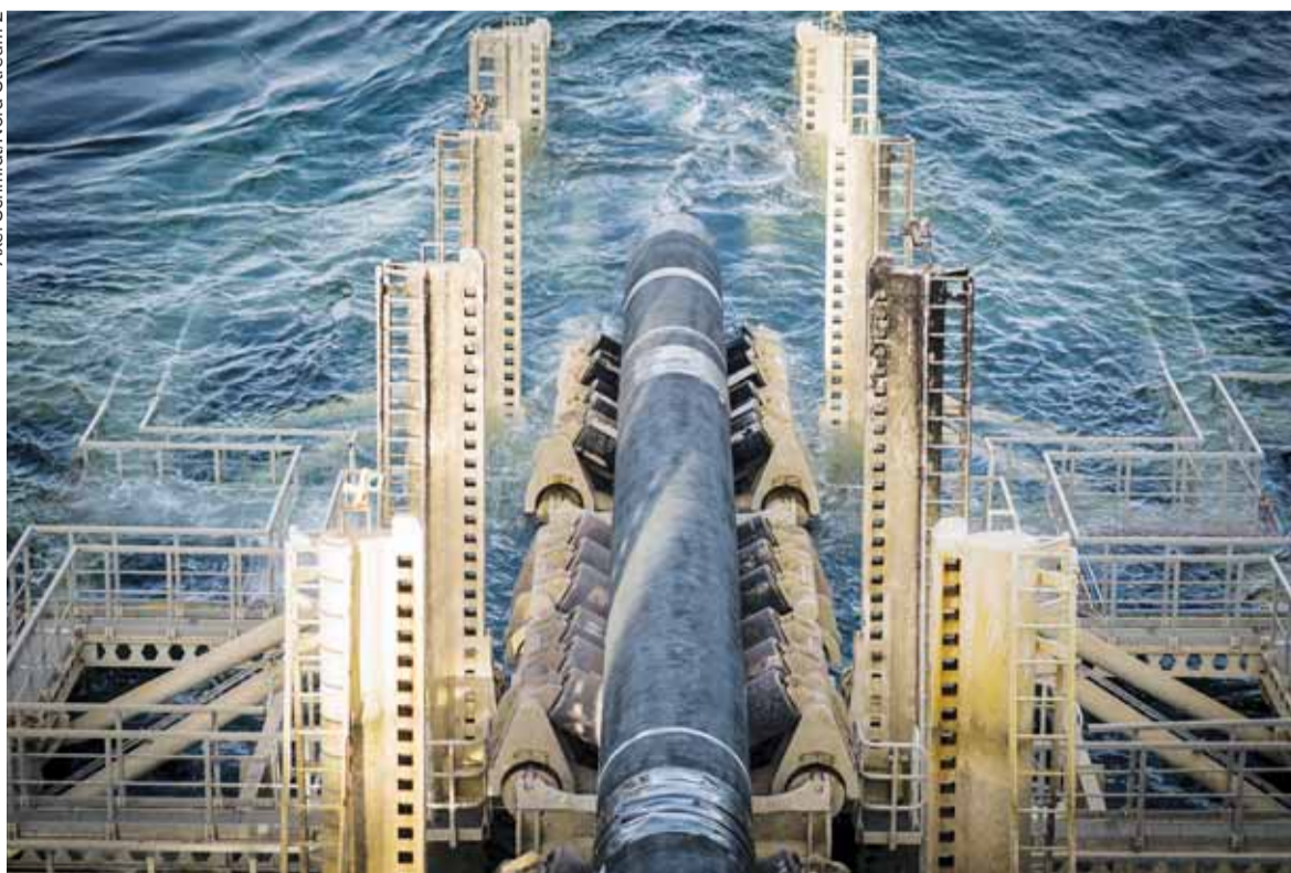
The Nord Stream 2 pipeline under construction by vessel Pioneering Spirit on Feb. 25, 2019. The $11 billion pipeline, which goes under the Baltic Sea to double the amount of natural gas transported annually from Russia to Europe to 110 billion cubic meters, has been under construction since 2015. For now, much of Russian gas goes to Europe through Ukraine's land-based gas transit system.
