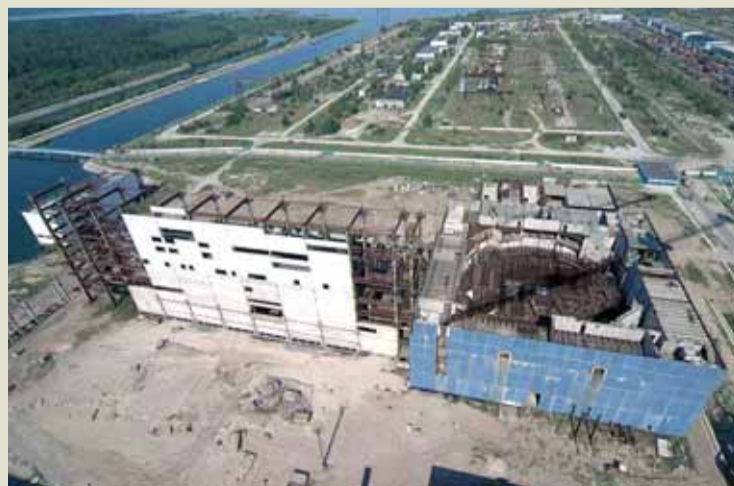
Units for a third and fourth reactor at the KhNPP have been left abandoned and exposed to the elements for years. (KhNPP)
