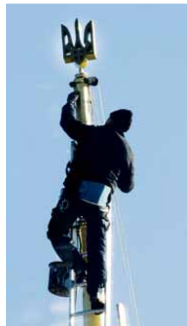
Worker installs Trident on the spire of the Verkhovna Rada in Kyiv on Oct. 29, 2015
