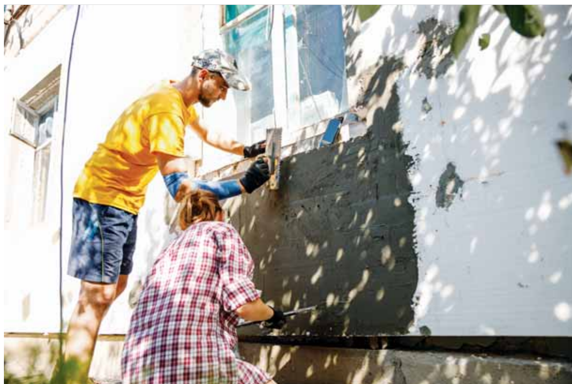
Participants of the volunteer program "Building Ukraine Together" ("Buduiemo Ukrainu Razom" – BUR) rebuild a house. Having started as an initiative to rebuild homes destroyed by Russia's war in the east, the volunteer organization now renovates abandoned areas and rebuild homes all across Ukraine.
