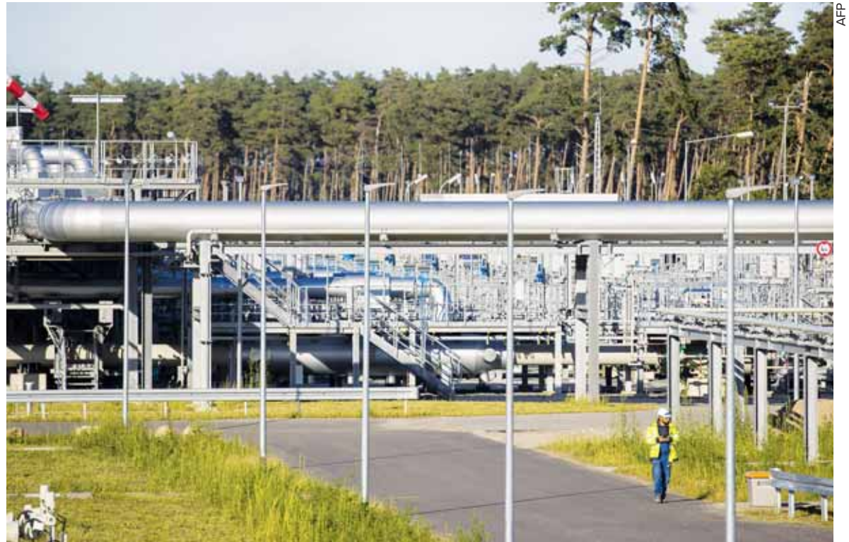
A worker walks by the Nord Stream 2 gas line landfall facility in Lubmin, north eastern Germany, on Sept. 7, 2020.
