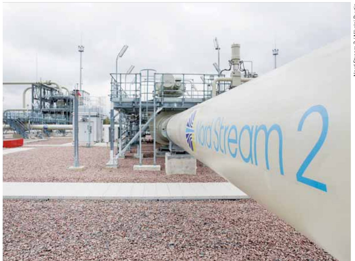
A Nord Stream 2 pipeline on Sept. 23, 2021 in Russia. The controversial pipeline completed in September will allow the Kremlin to send gas to Europe through the Baltic Sea and Germany instead of Ukraine, potentially causing at least $1.5 billion in lost transit fees. Kyiv is turning to Ankara to develop its energy security, but Turkey has its own agenda with Russia.
