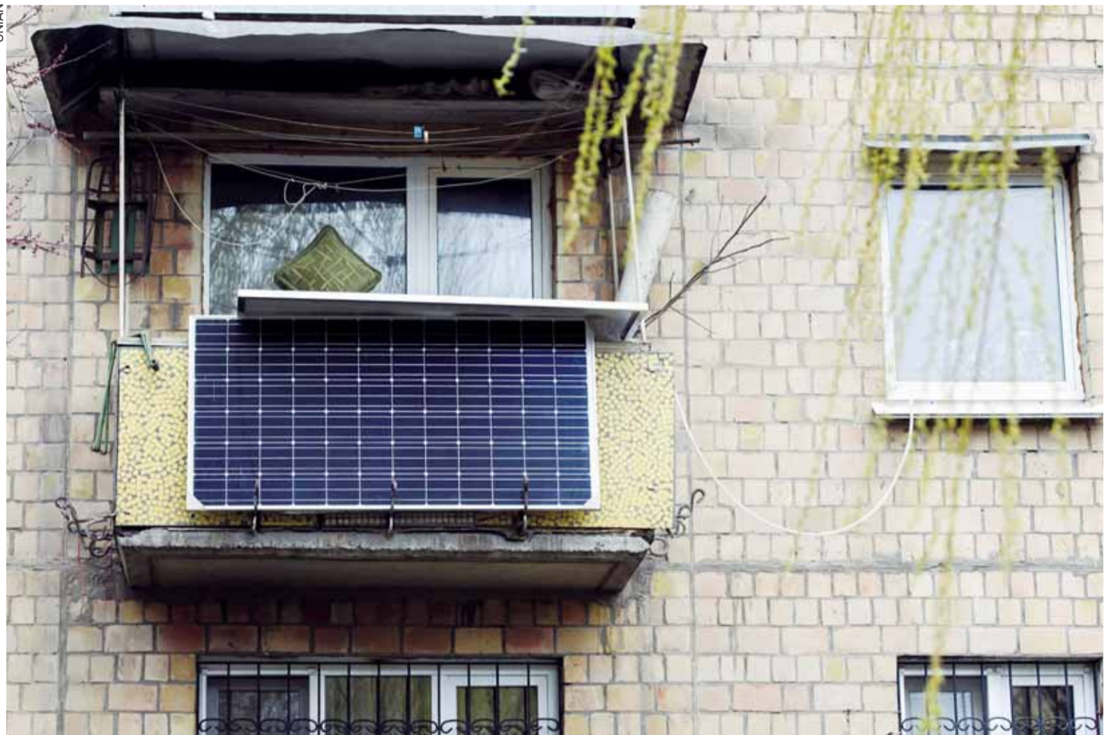
A solar panel installed on a balcony of an apartment building in Kyiv on March 31, 2020. Over 27,500 Ukrainian households have installed solar panels at home as of October 2020, with a general capacity of 712 megawatts.
