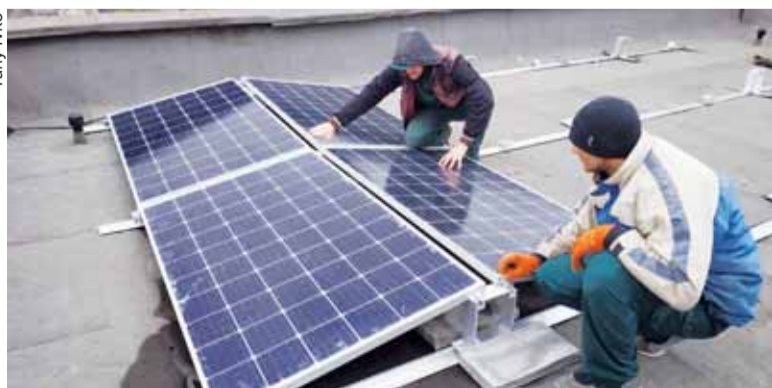
Workers install solar panels on the roof of a 4,000-square-meter apartment building in the Troieshchyna district in Kyiv. Local firm Avrora Term has invested $330,000 in the solar panels on this roof and expects to return the investment in six years.
