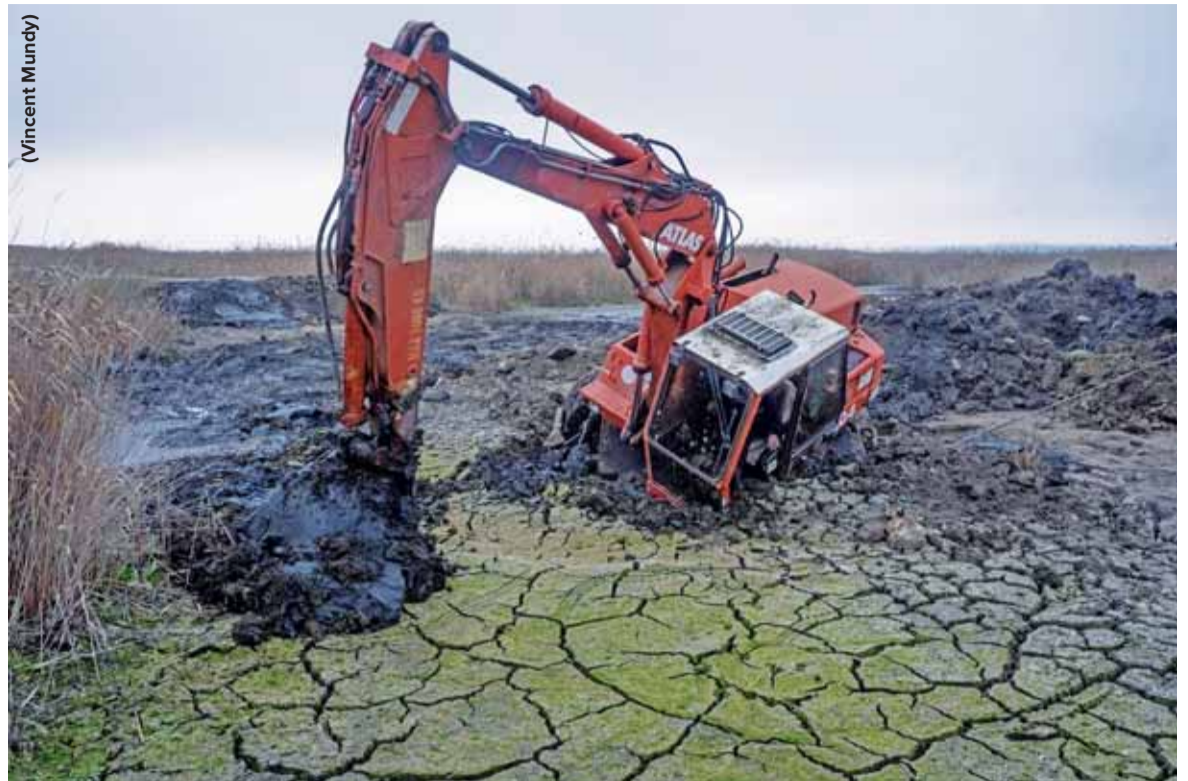
An excavator machine used to remove an obsolete river dam is partially consumed in a degraded area of wetland beside the Kohlynyk river within the territory of the Danube Biosphere Reserve (DBR) near Tatarbunary.
