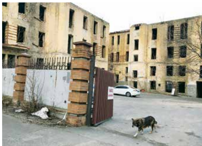
Hit by fire in 2003, the century-old building at 50 Velyka Vasylykivska is gradually falling apart. Historian Olena Mokrousova says prominent Kyiv architect Joseph Zekzer designed the house. (Kostyantyn Chernichkin)
