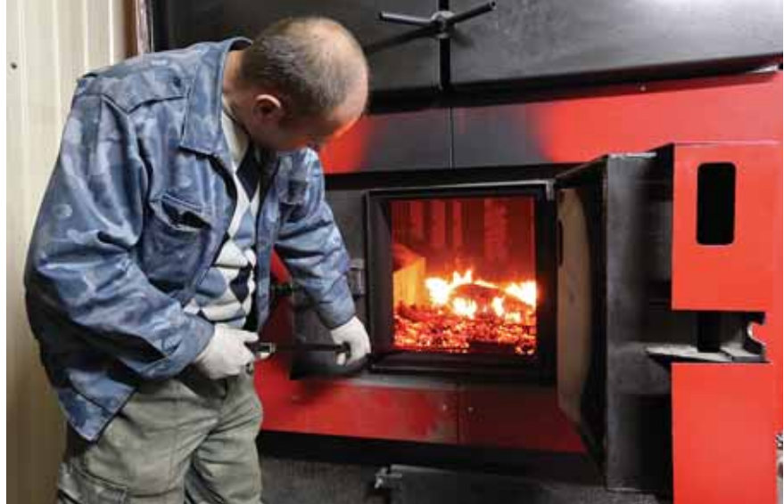
A stoker moves wood pellets in a solid fuel-boiler in maternity hospital No. 5 in Kyiv on Nov. 24. Alternative energy company Ukrteplo installed the solid fuel boiler and supplies the hospital with pellets. (Volodymyr Petrov).
