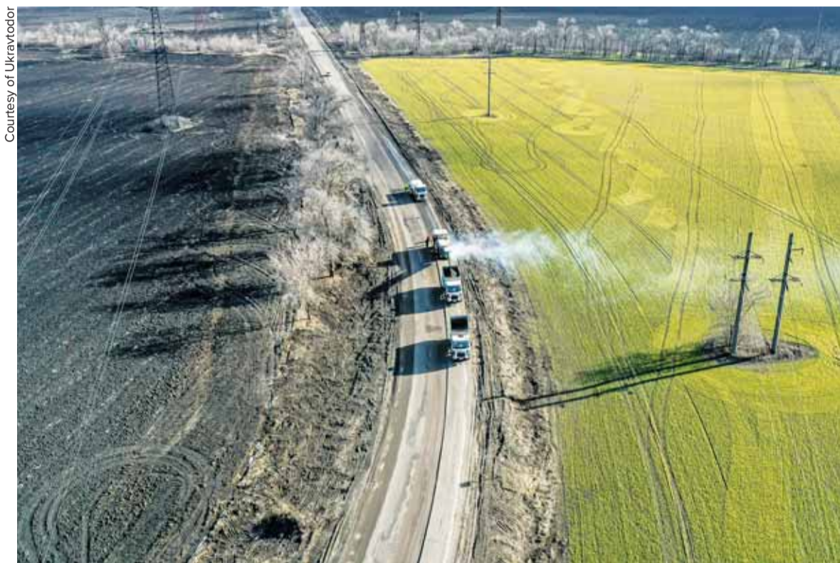
Workers begin reconstruction of a 10-kilometer section of a road in Zaporizhia Oblast on March 11. As part of President Volodymyr Zelensky's large-scale infrastructure program known as Big Construction, state road agency Ukravtodor plans to repair all 255 kilometers of the Kropyvnytsky–Kryvyi Rih–Zaporizhia N-23 highway in 2021.
